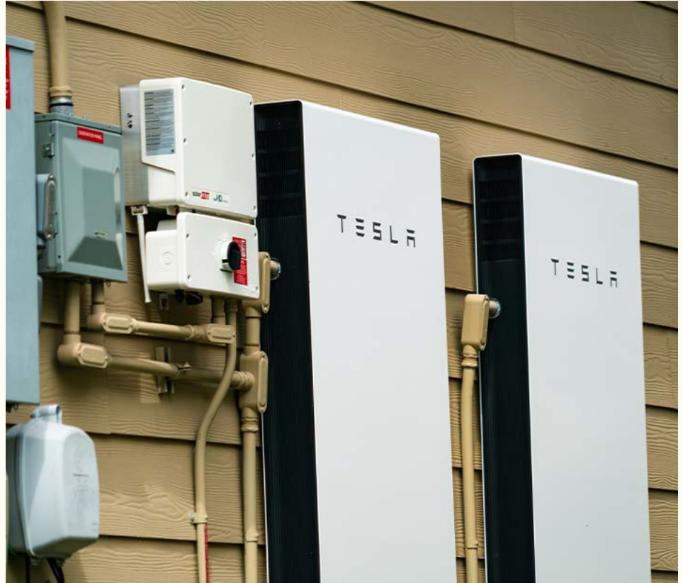
Tesla Powerwall batteries | Shutterstock
